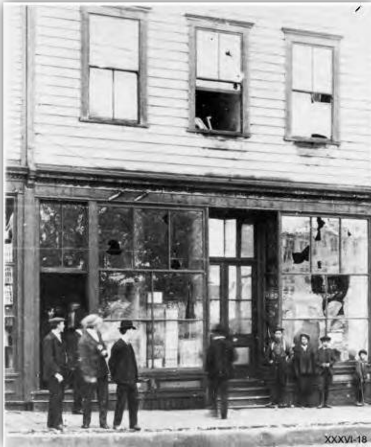
“Building damaged during Vancouver riot of 1907 - 124 Powell Street, $78,” photograph, 1907, JCPC 36.018, Japanese Canadian Research Collection, University of British Columbia Library Rare Books and Special Collections, Vancouver, Canada. Reproduced with permission.
